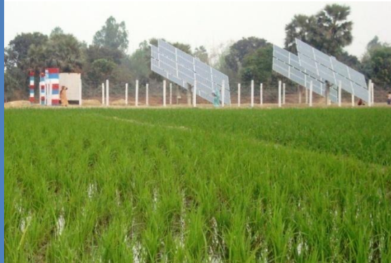
11.2 KW solar irrigation pump project at Sapahar, Naogaon
