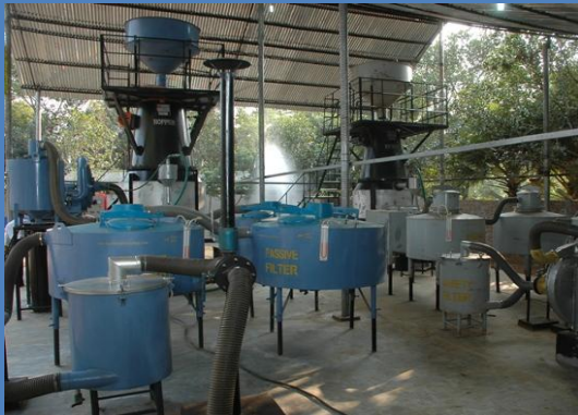
250 KW biomass gasification based power plant
