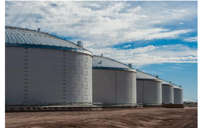
Molten-salt storage tanks at Solana CSP plant in Arizona. Credit: Abengoa
