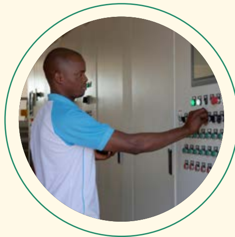
Control room of the Magula Pumping Station (Baixo Limpopo Irrigation Scheme, Gaza)
