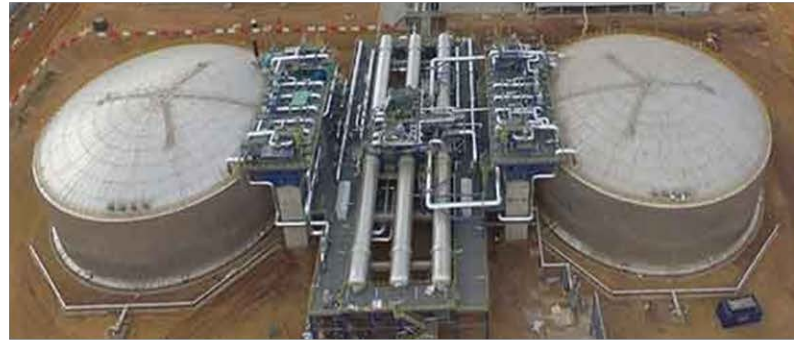
Molten salt tanks – hot and cold
