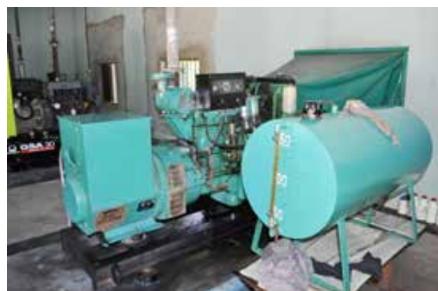
A diesel generator installed at a powerhouse
