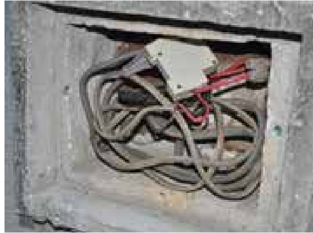
Distribution box at an island
