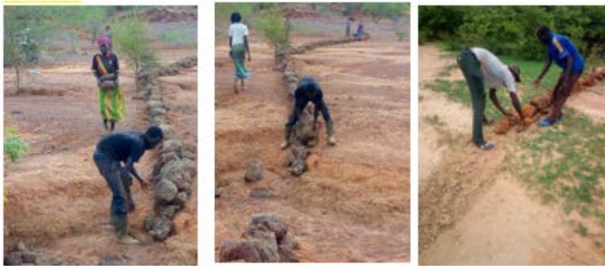
In Burkina Faso, communities have learned how to lay stone barriers along contour lines to improve degraded land.
