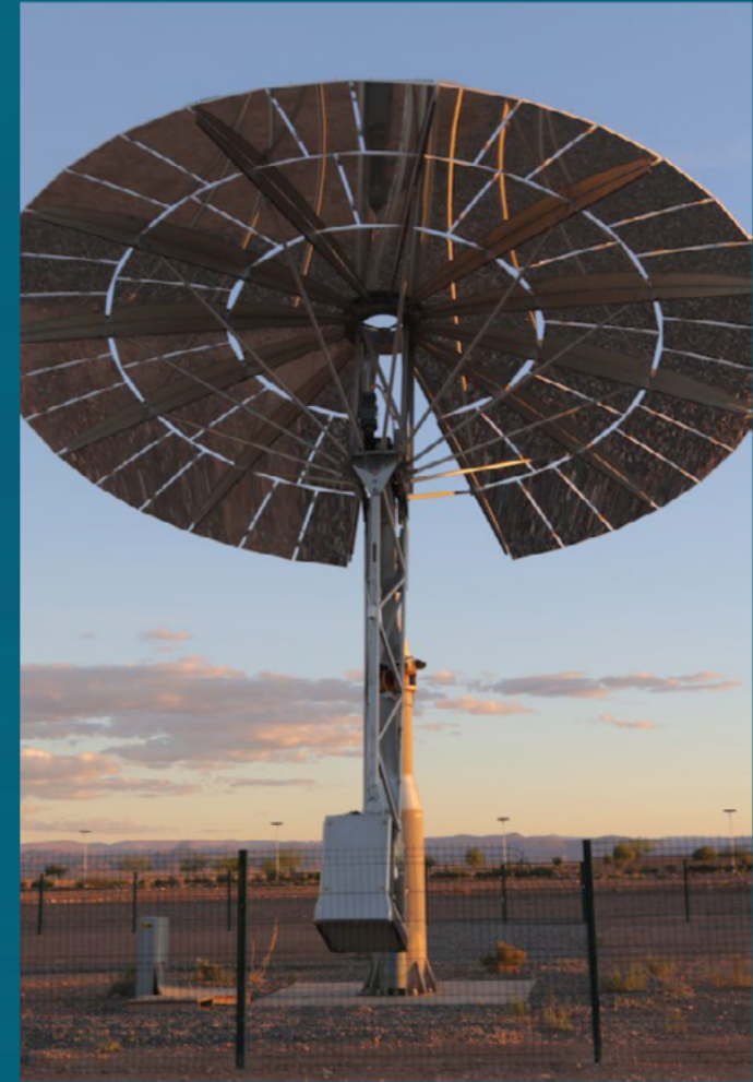
Noor Concentraed Solar Power Plant, Morocco. Source: CIF Flicker
